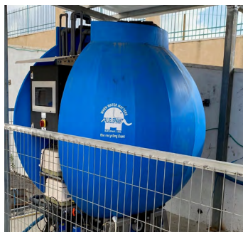
BluElephant decentralized wastewater units WOP Palestinian Water Authority
