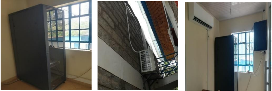
Figure 6: Well and safely installed servers and at controlled room temperature rating
